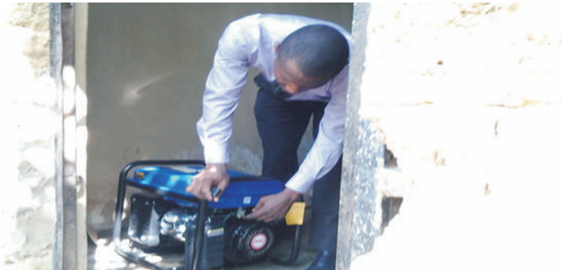
Figure 3: Generator with switch on and empty fuel tank at the house under investigation in Akure, 2014
